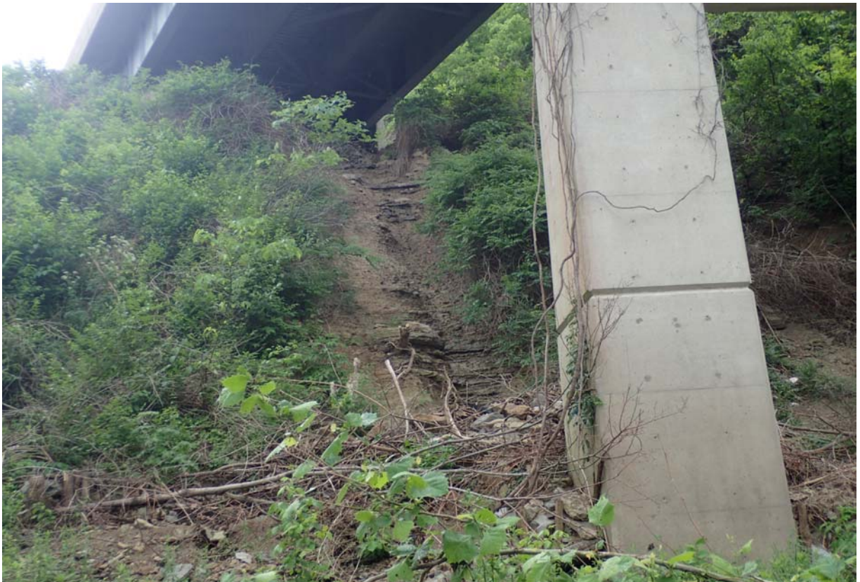
View of a significant erosion gulley in span 3.
