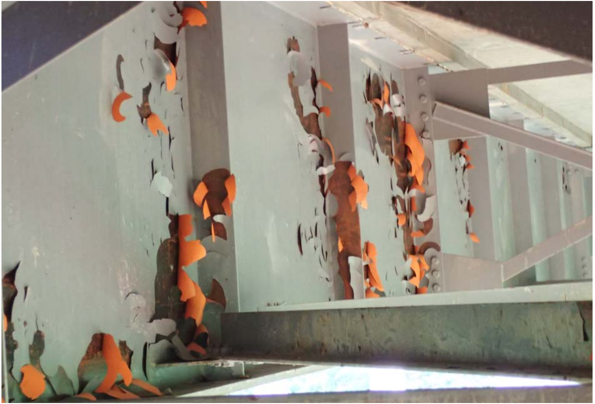
View of several large areas of flaking/peeling paint on the south face of girder 3 from the south in span 1.
