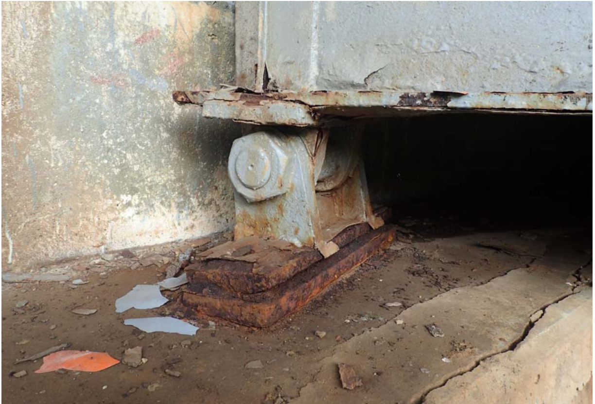
View of the south bearing at abutment 1. Notice the moderate to heavy corrosion in the lower rocker and masonry plate. Both anchor bolts are missing.
