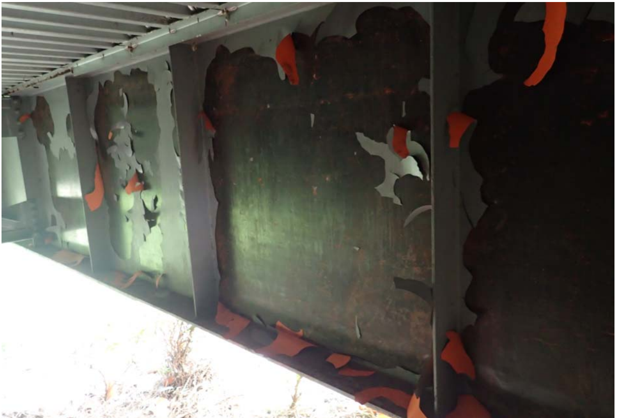
View of large areas of paint failure on the interior face of the north girder near abutment 4.
