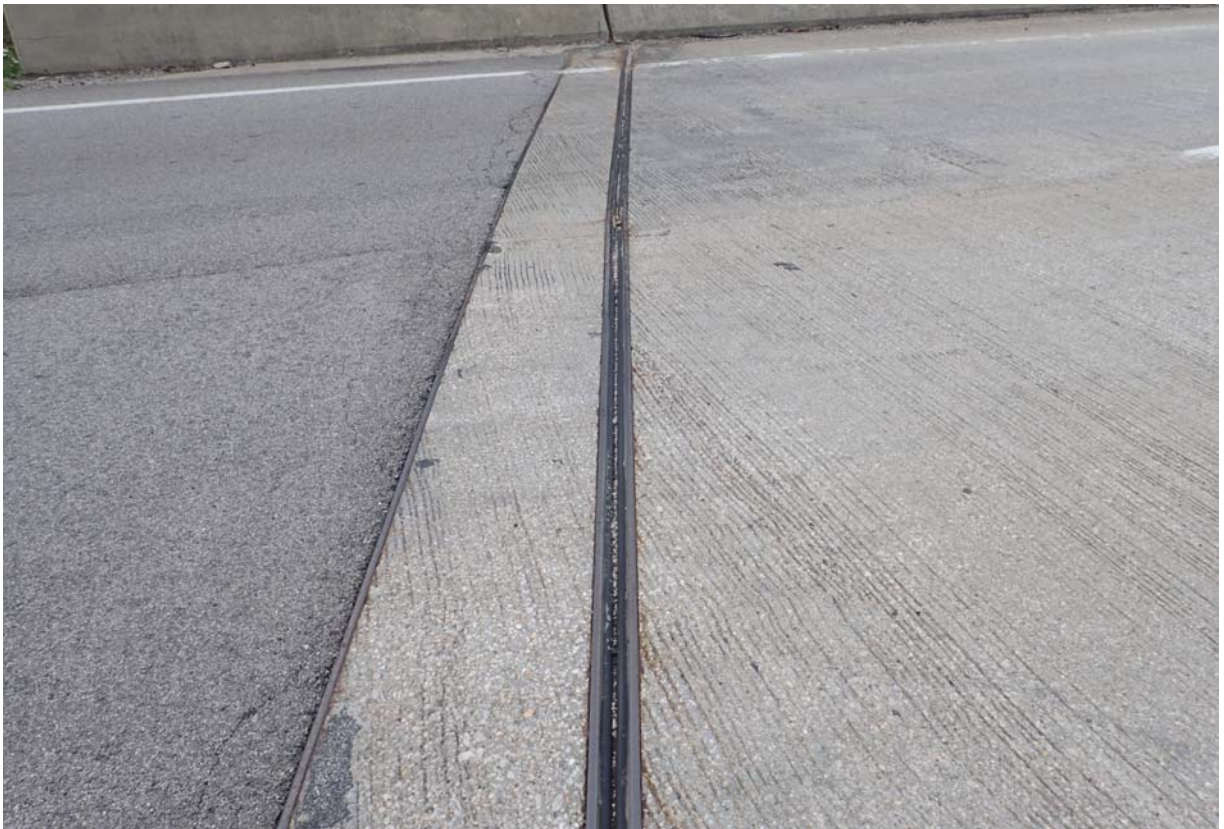
View of the transverse joint at abutment 4. It is partially full of debris and has some small tears.
