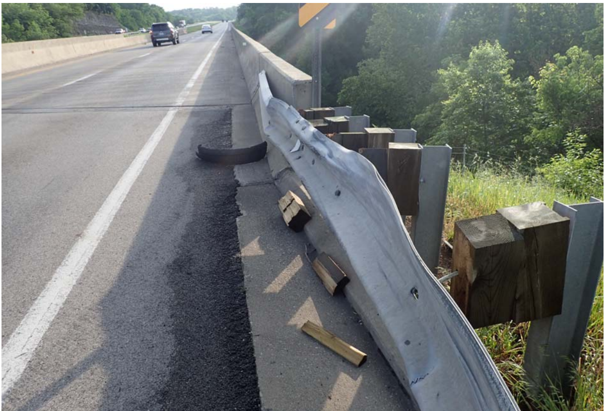
View of impact damage to the south approach railing at abutment 1.
