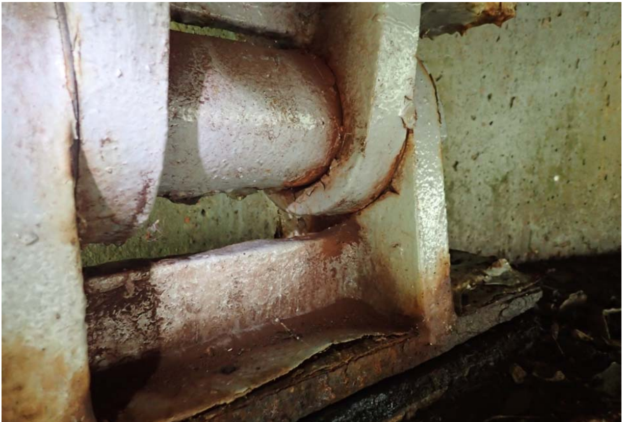
View of bearing 2 from the south at abutment 1. Notice the fretting.
