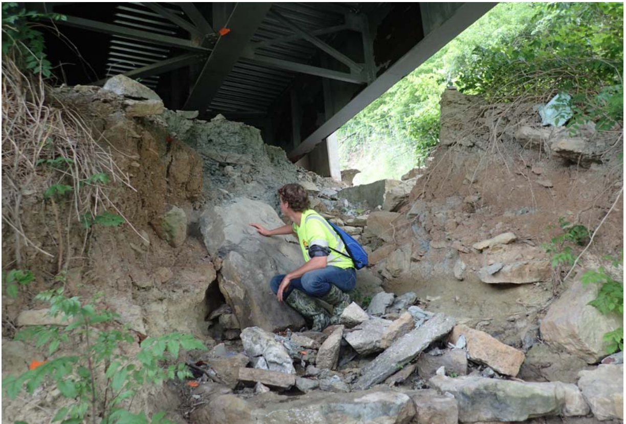
View of a significant erosion gulley in span 3 in front of abutment 4.
