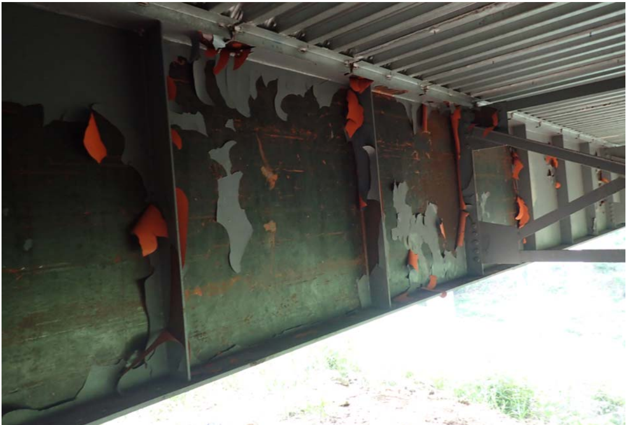
View of large widespread areas of flaking/peeling paint on the south face of the north girder in span 1.
