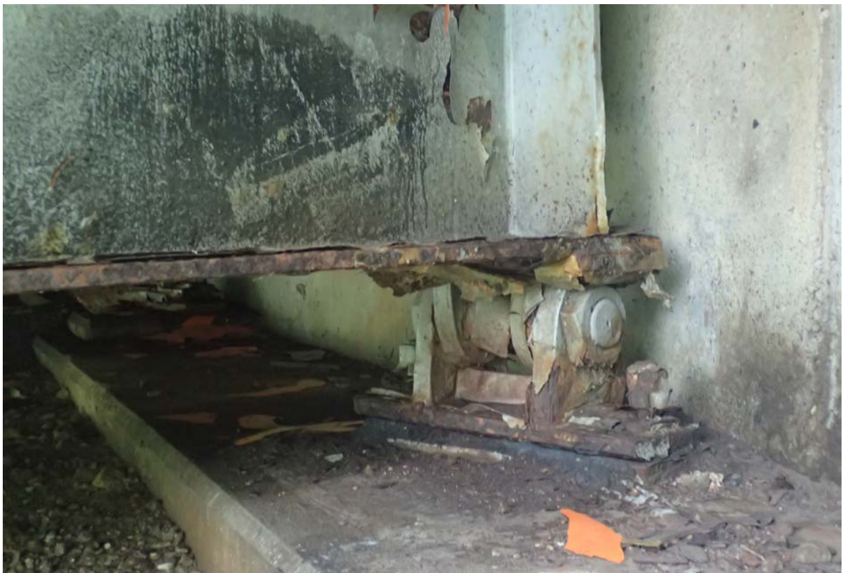
View of the south bearing of abutment 4. Notice the moderate to heavy corrosion in the lower portions of the bearing. Notice the flaking paint and corrosion along the bottom flange of the girder.
