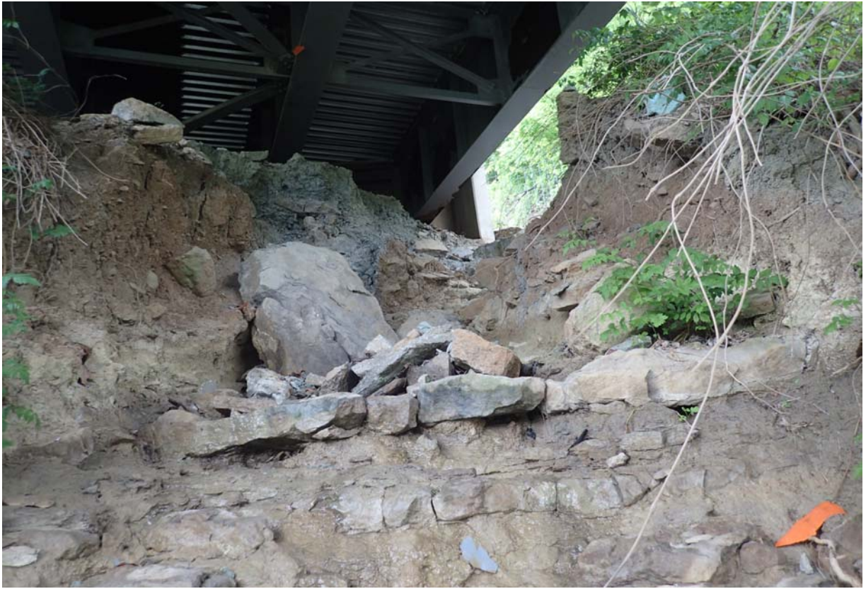
View of a significant erosion gulley in span 3 in front of abutment 4.
