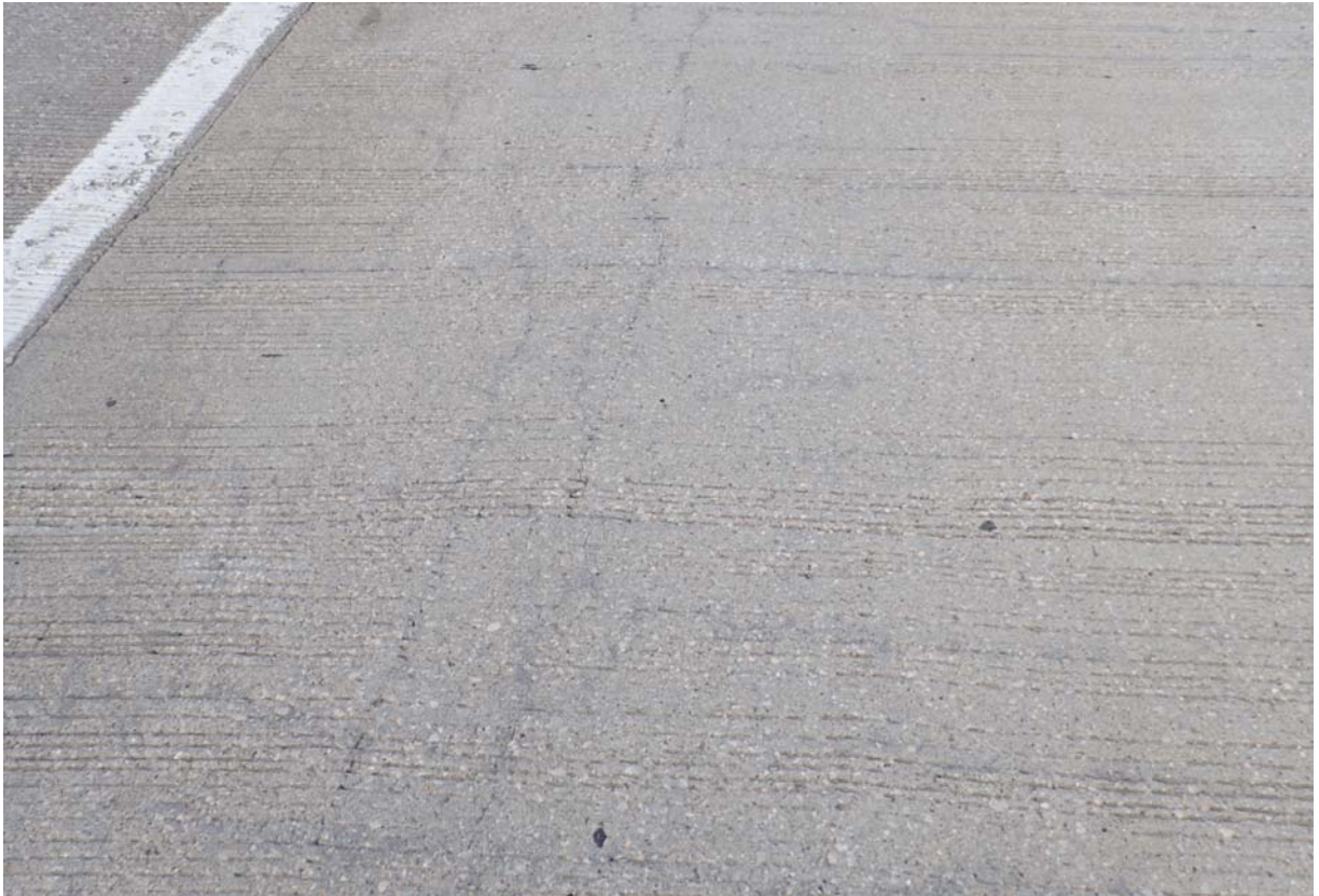
Typical view of some minor sized longitudinal cracking in the left lane.
