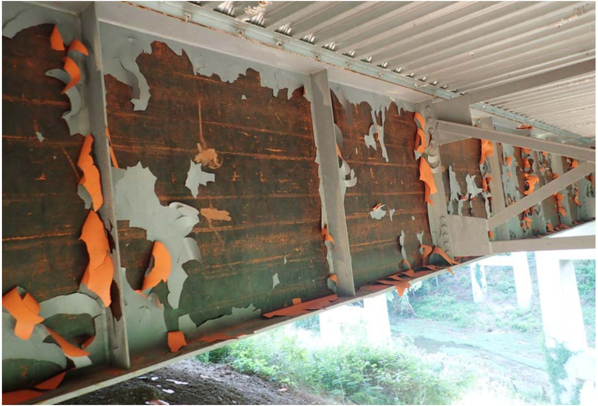
View of large widespread areas of flaking/peeling paint on the south face of girder 2 from the south in span 1.
