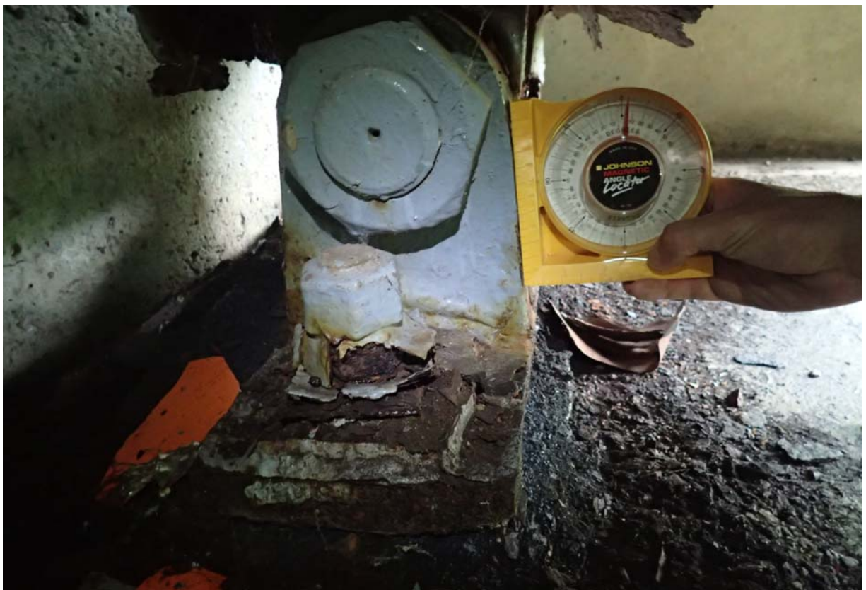
View of the south bearing at abutment 4. It is tilted toward the backwall ~ 6 degrees. The measurement was taken on a tapered surface so the actual rotation is a little less.
