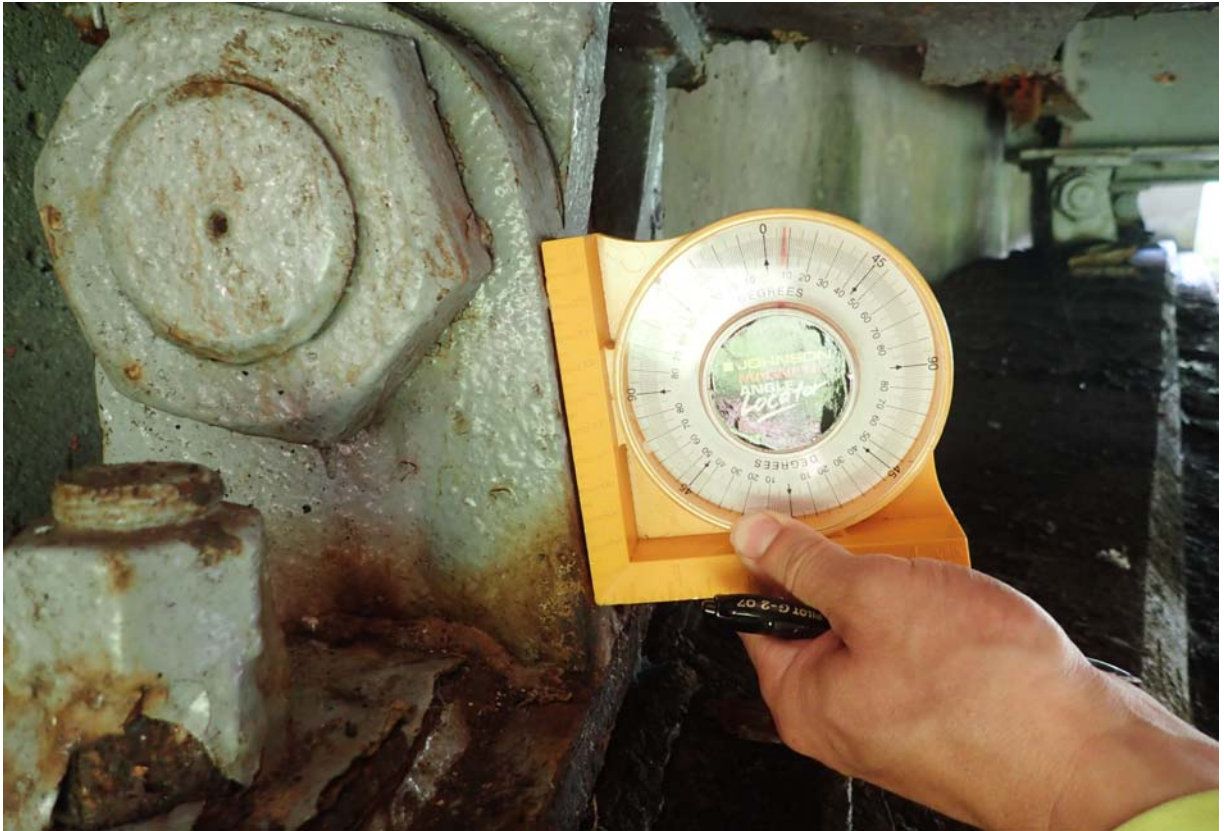
View of bearing 2 from the south at abutment 1. It is tilted toward the backwall ~ 9 degrees. The measurement was taken on a tapered surface so the actual rotation is a little less.
