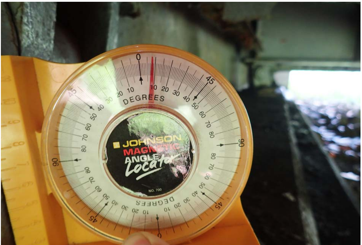
View of bearing 2 from the south at abutment 1 tilted toward the backwall ~ 9 degrees. The measurement was taken on a tapered surface so the actual rotation is a little less.
