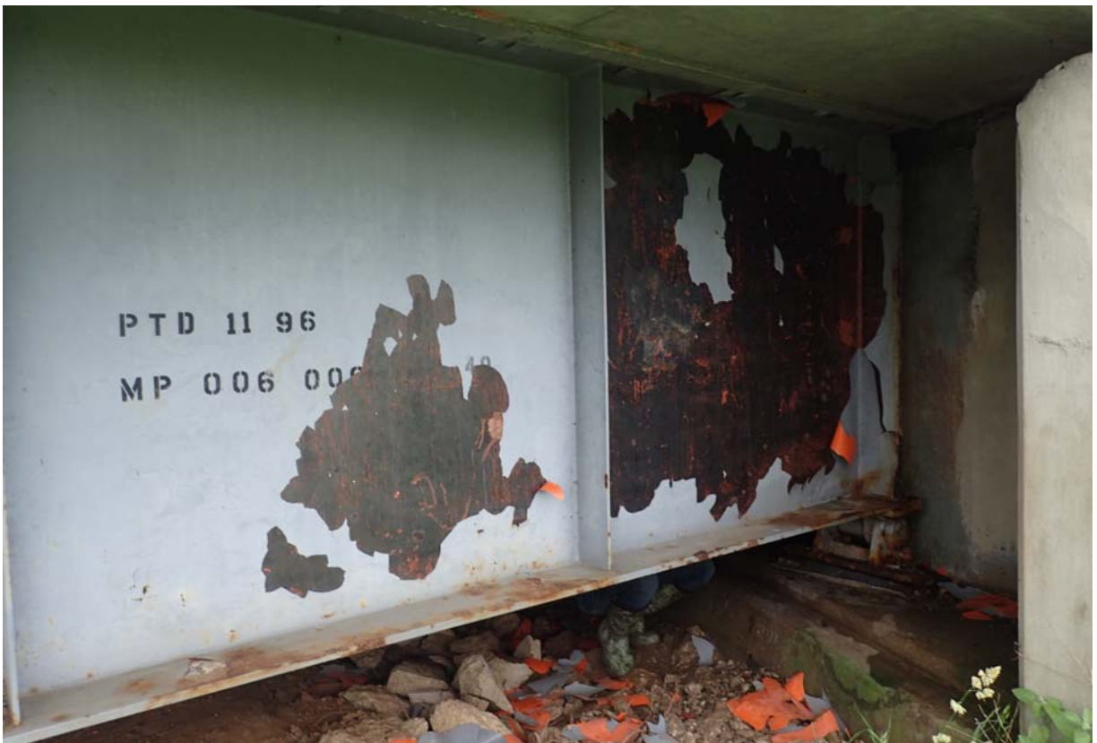
View of a large area of paint failure on the exterior face of the north girder at abutment 1.
