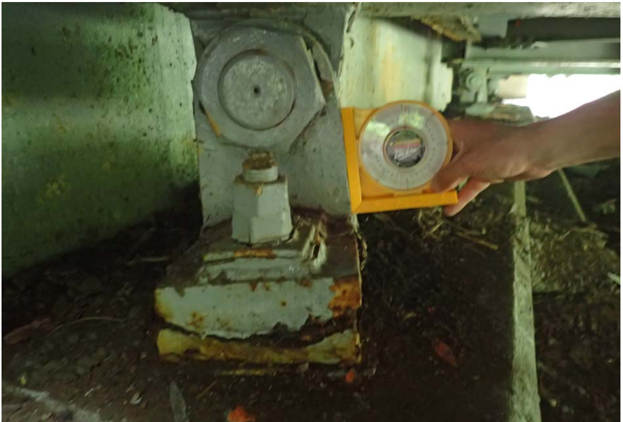
View of bearing 3 from the south at abutment 4. It is tilted toward the backwall ~ 6 degrees. The measurement was taken on a tapered surface so the actual rotation is a little less.
