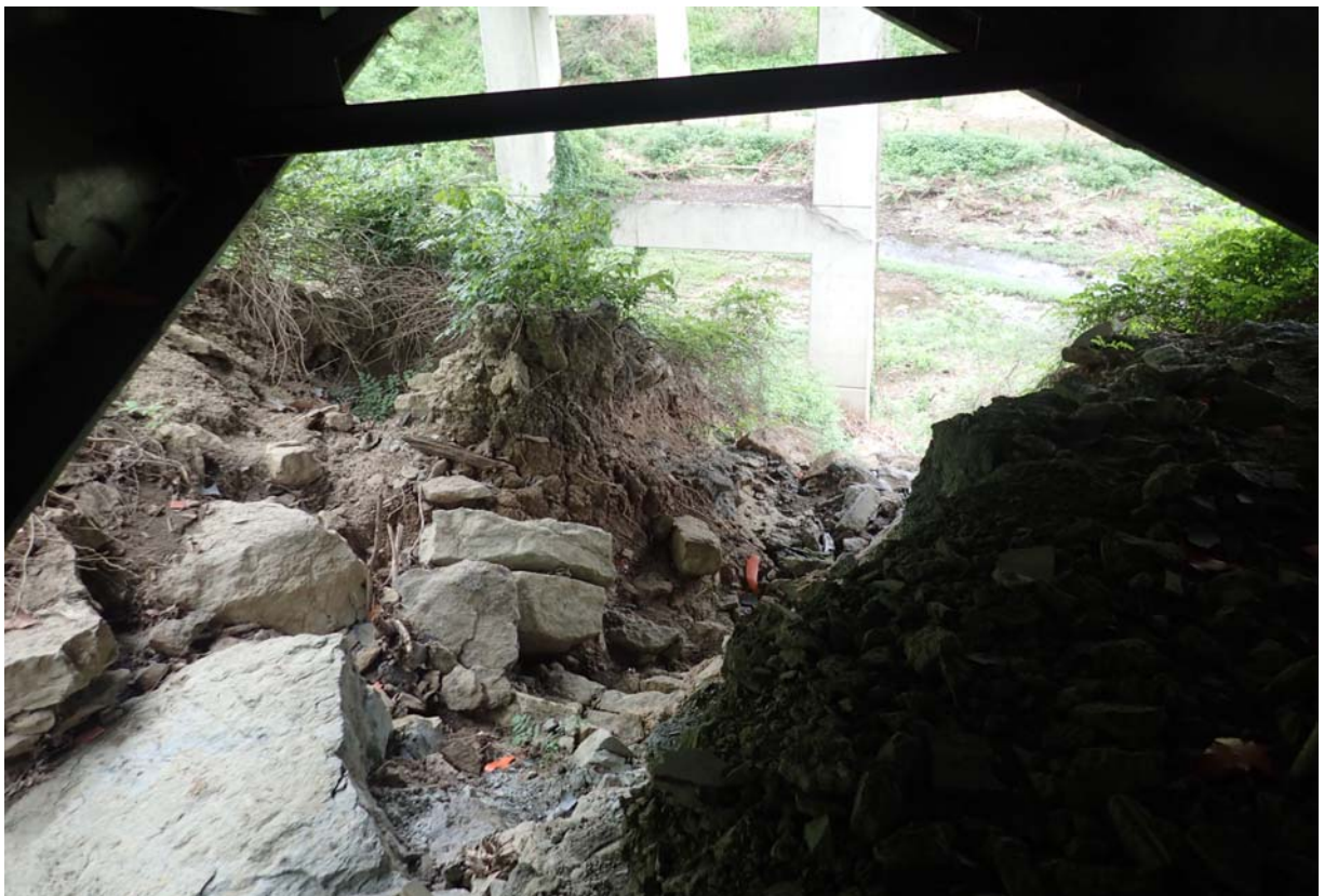
View of a significant erosion gully in span 3 at the south end of abutment 4.
