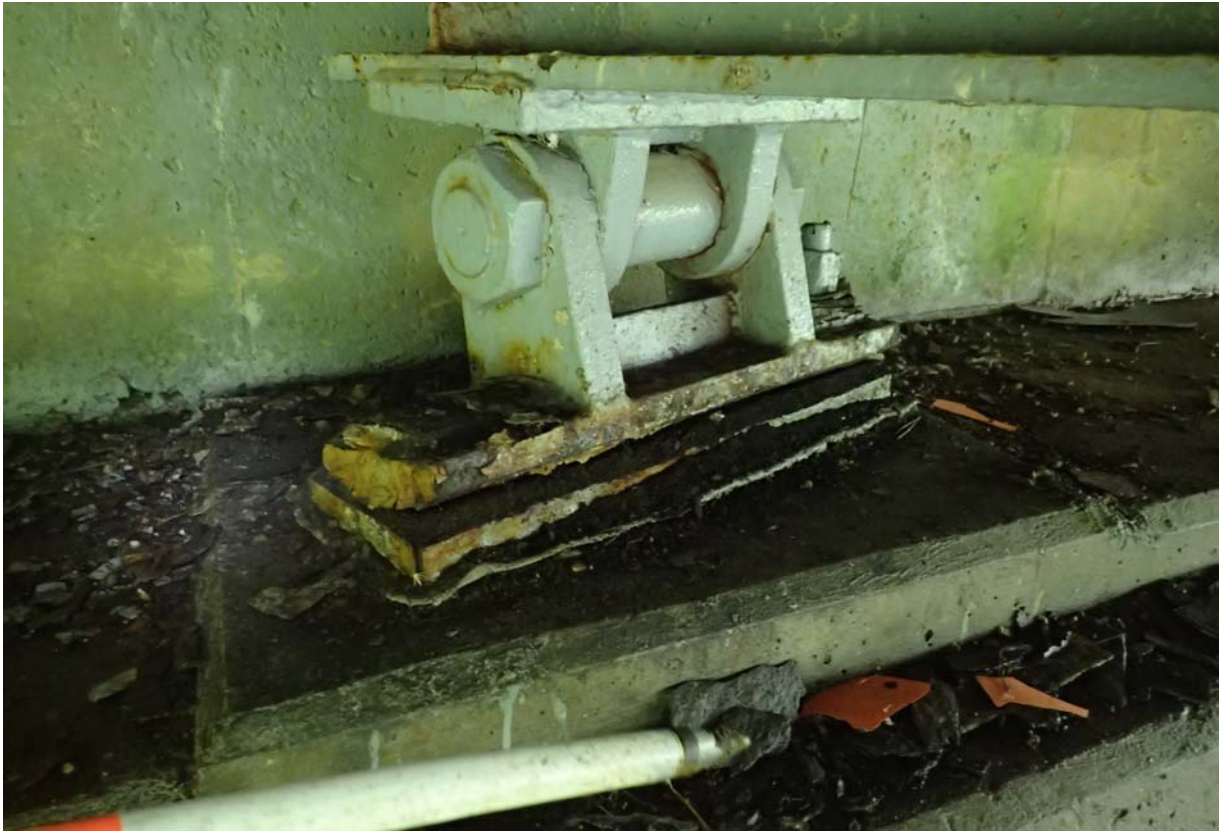
View of bearing 3 from the south at abutment 1. It is missing the south anchor bolt and is tilted toward the backwall ~ 16 degrees. The measurement was taken on a tapered surface so the actual rotation is a little less.
