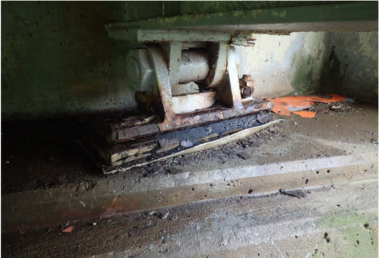
View of the north bearing at abutment 1. Notice the moderate to heavy corrosion. It is missing the south anchor bolt and is tilted toward the backwall ~ 19 degrees. The measurement was taken on a tapered surface so the actual rotation is a little less.
