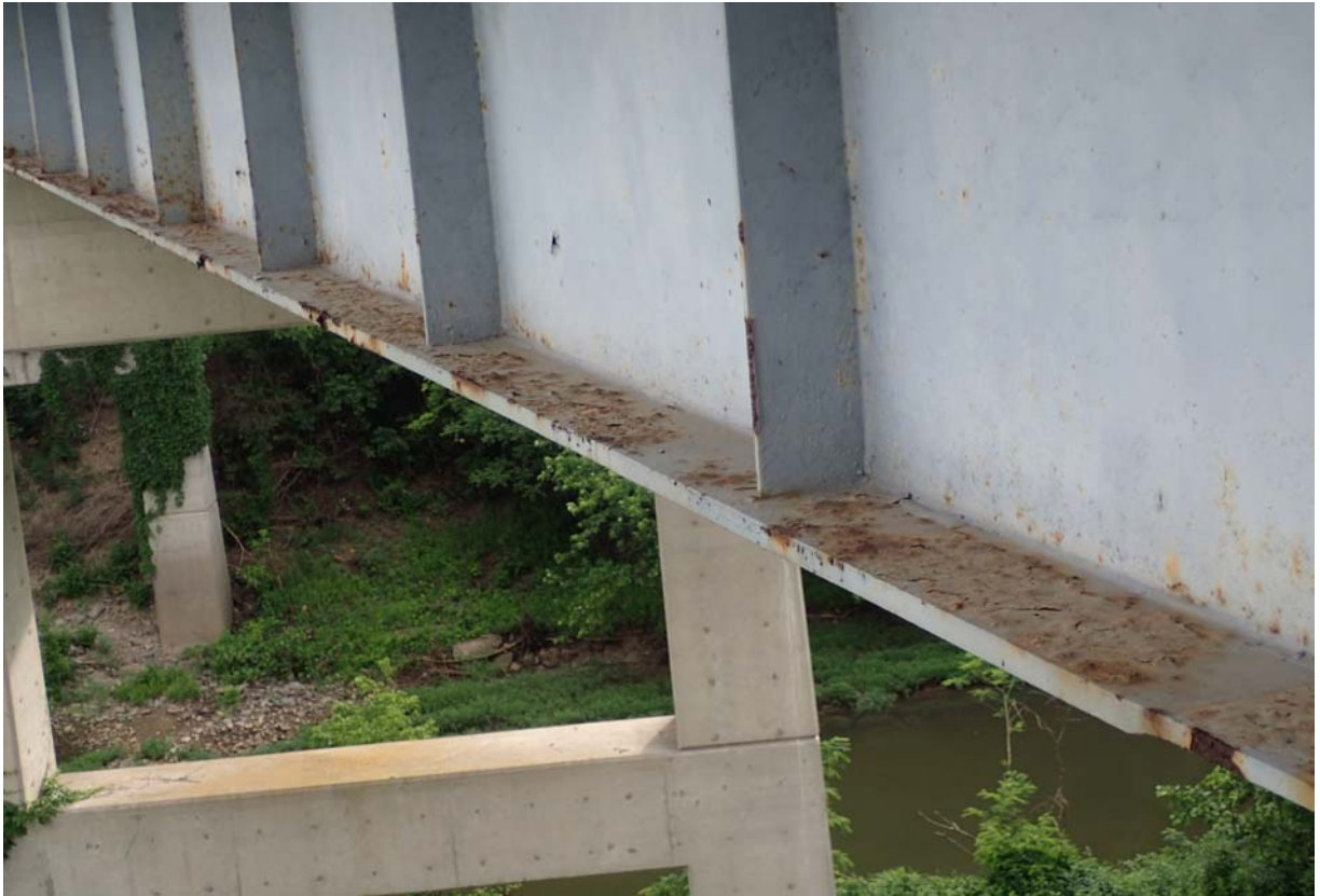
View of bubbling paint along the top of the exterior bottom flange of the north girder in span 1.
