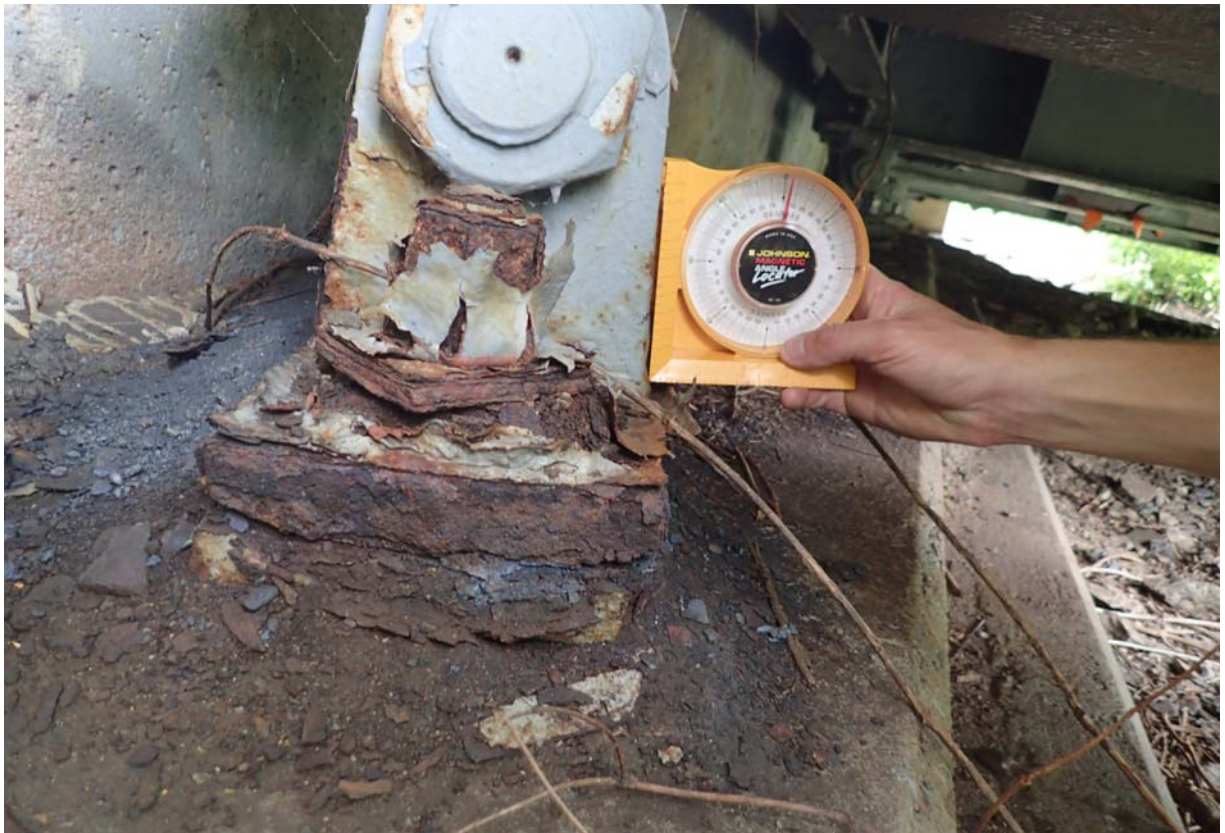
View of the north bearing at abutment 4. Notice the heavy corrosion in the lower rocker and masonry plate. It is tilted toward the backwall ~ 6 degrees. The measurement was taken on a tapered surface so the actual rotation is a little less.
