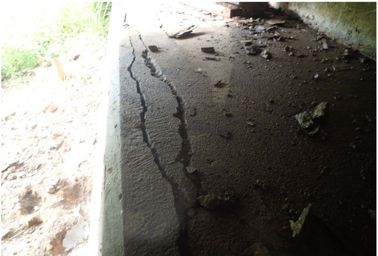
View of up to a 1/2" wide horizontal crack in the top south end of abutment 1s breastwall.
