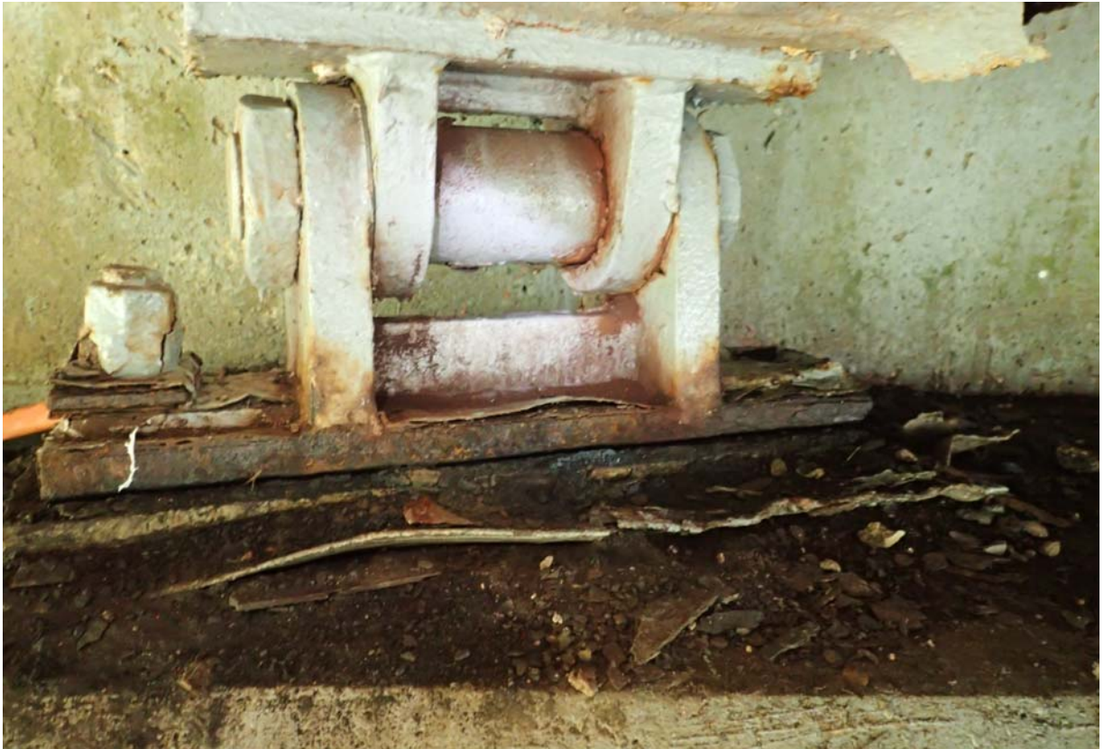
View of bearing 2 from the south at abutment 1. Notice the fretting, moderate to heavy corrosion, and the north anchor bolt is missing.
