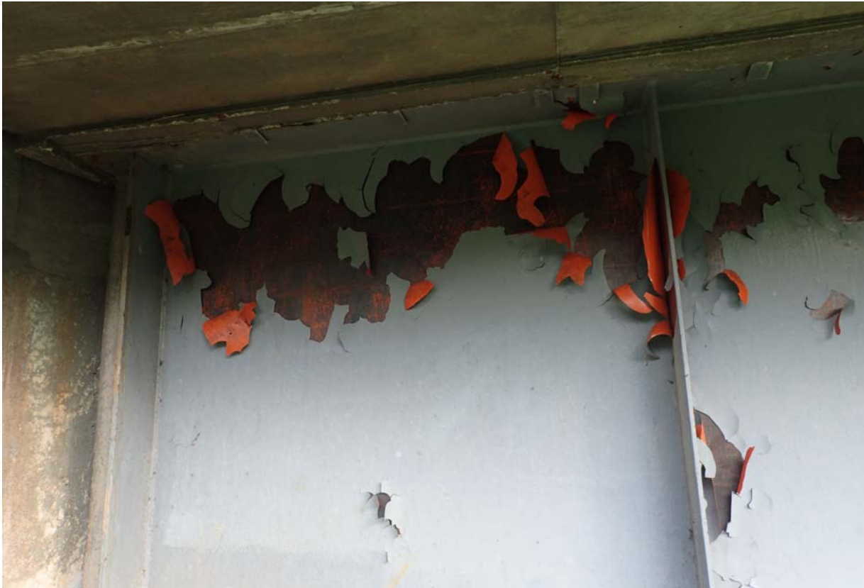
View of a large area of flaking/peeling paint on the exterior face of the south girder
