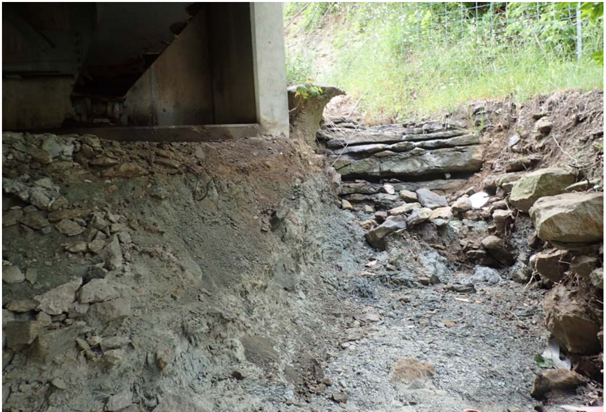
View of a significant erosion gulley in span 3 at the south end of abutment 4.
