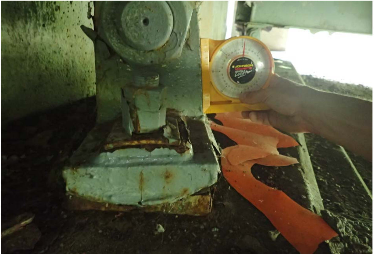
View of bearing 2 from the south at abutment 4. It is tilted toward the backwall ~ 6 degrees. The measurement was taken on a tapered surface so the actual rotation is a little less.
