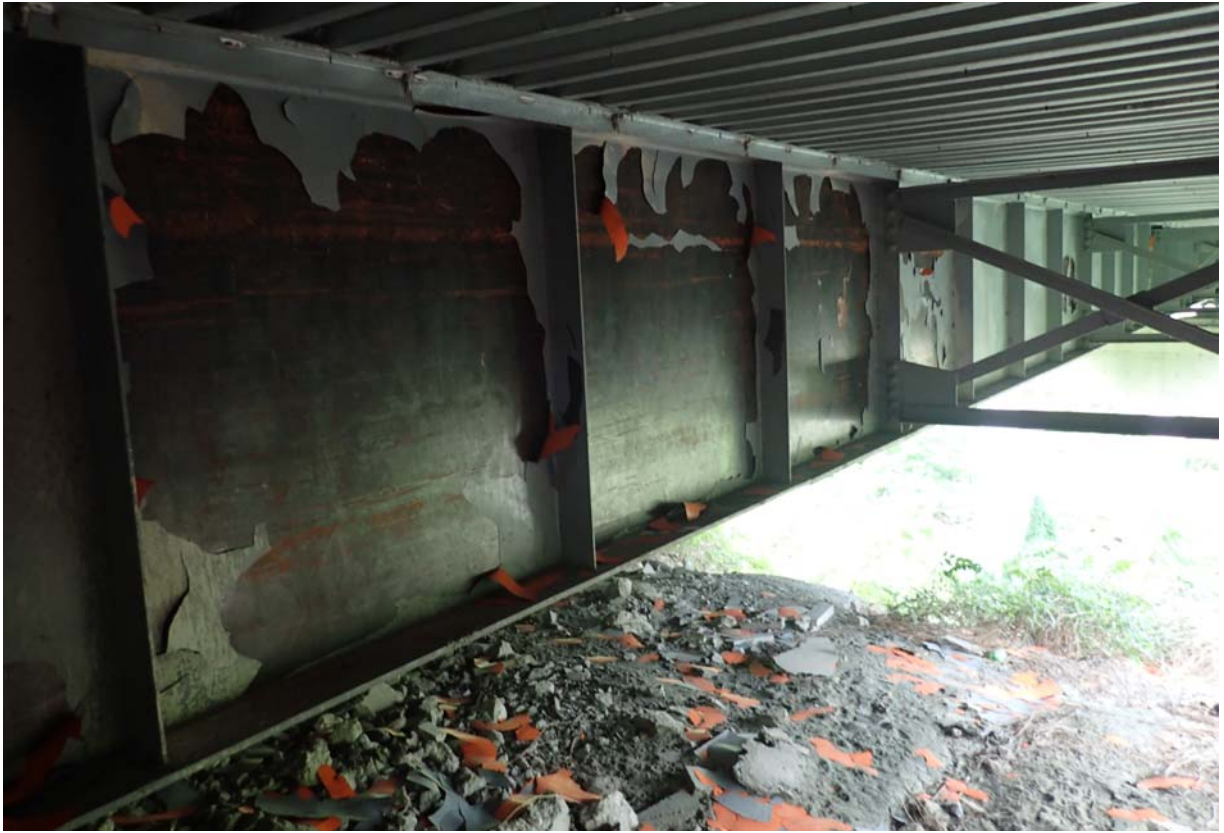
View of large areas of paint failure on girder 3 from the south near abutment 4.
