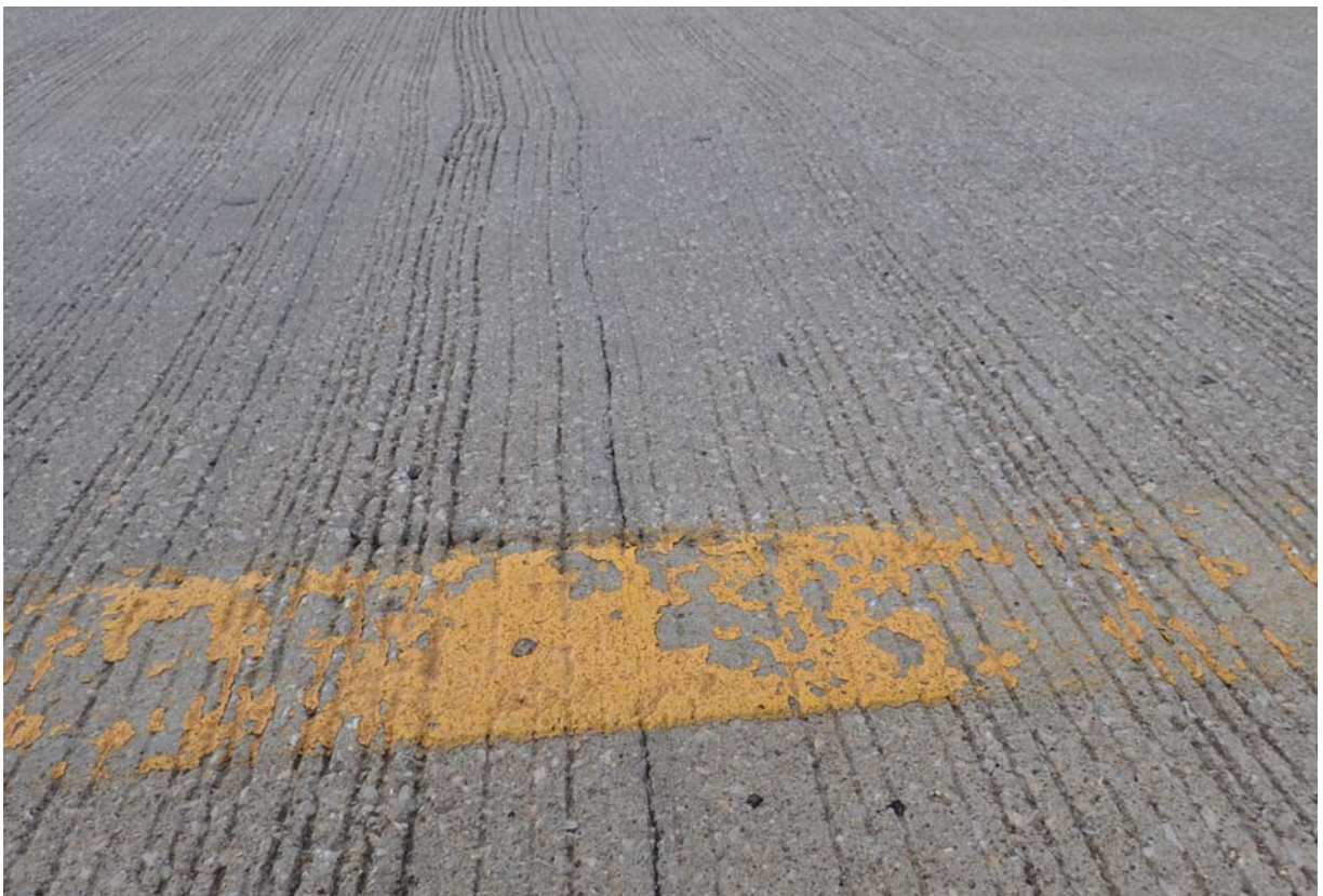
View of a minor sized transverse crack in the wearing surface in span 2 near midspan.
