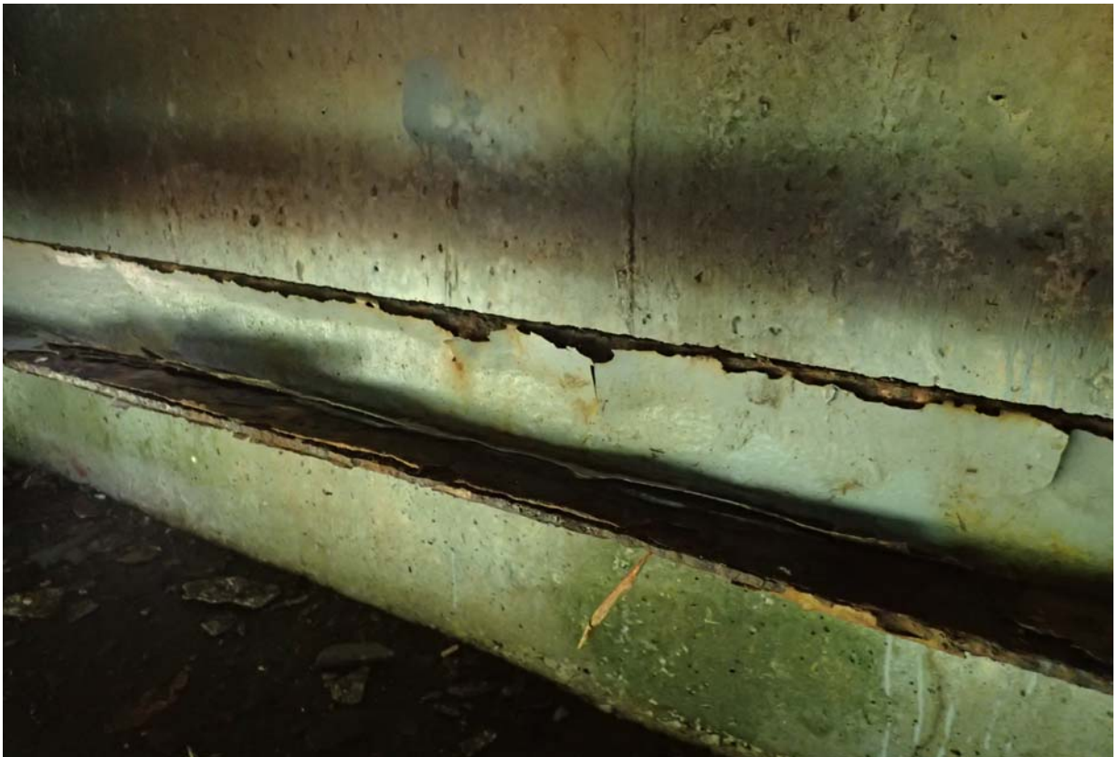
View of flaking paint with heavy corrosion and pitting of the lower angle of the cross bracing of the diaphragm between girders 2 and 3 from the south at abutment 1.
