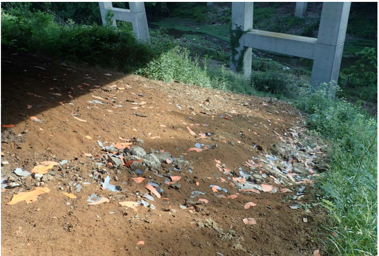
View of a large amount of flaking/peeling paint along the embankment in front of abutment 1.
